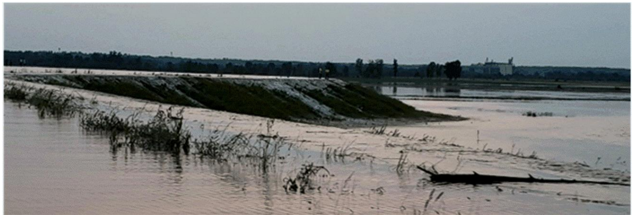
Figure 3.2 Levee overtopping leading to non-breach (Source: USACE Rock Island District 2019 Mississippi River Flood Fight digital photo library)
